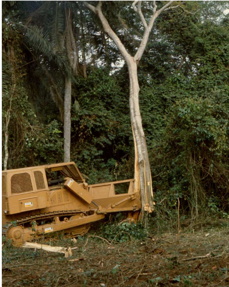
Fig. 2. Deforestation of tropical rainforest in southern Nigeria. The rate of tropical deforestation may be 20 million hectares per year.
